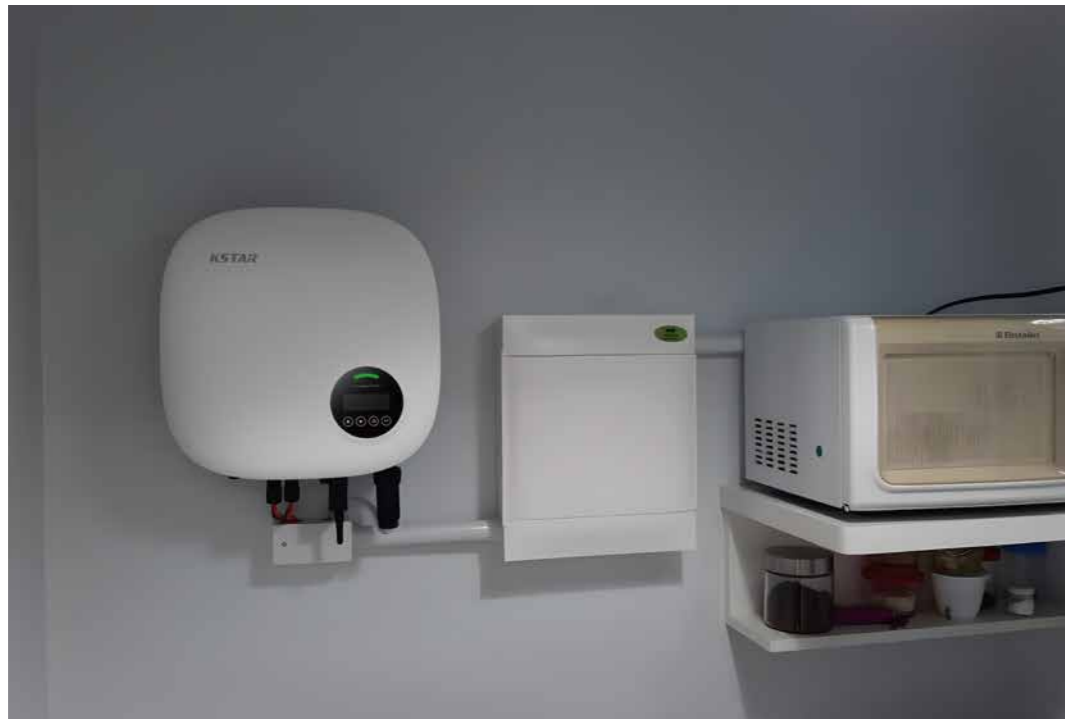
10 Residential Solar Project in Brazil
