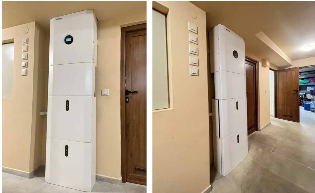
03 Residential ESS Project in Bulgaria
