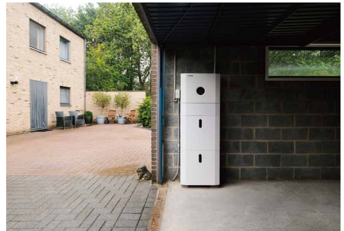
11 Residential ESS Project in Belgium
