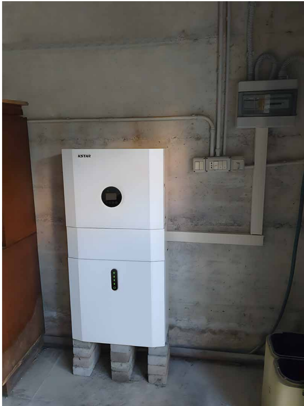
01 Residential ESS Project in Italy
