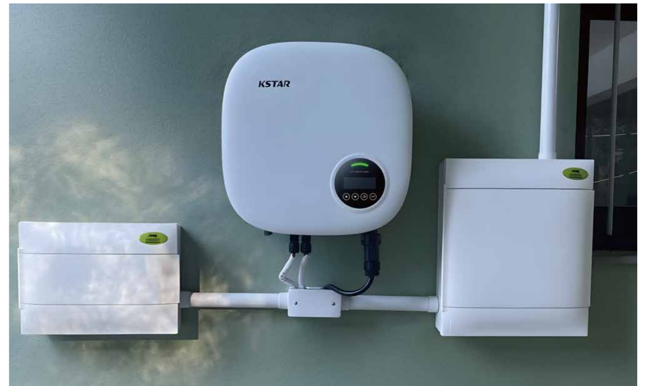
07 Residential Solar Project in Brazil
