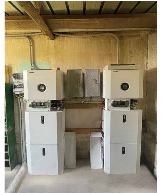
05 Residential ESS Project in Italy
