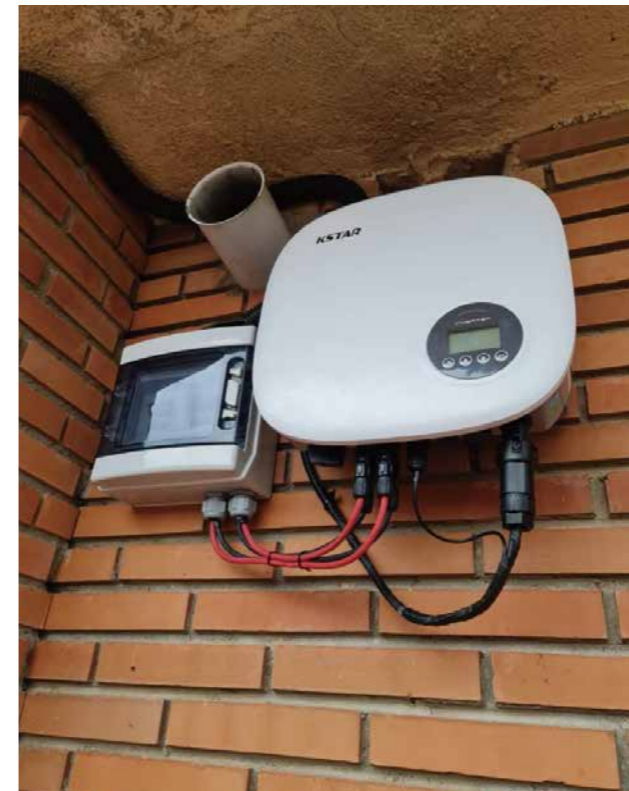
04 Residential Solar Project in Brazil
